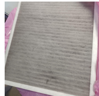
IMAGE 4: Air Filter removed showing Dust
