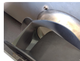
IMAGE 6: Clean Air compartment with no wear or dust visible
